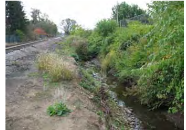
Highly Eroded Side Slopes along Whites Run
